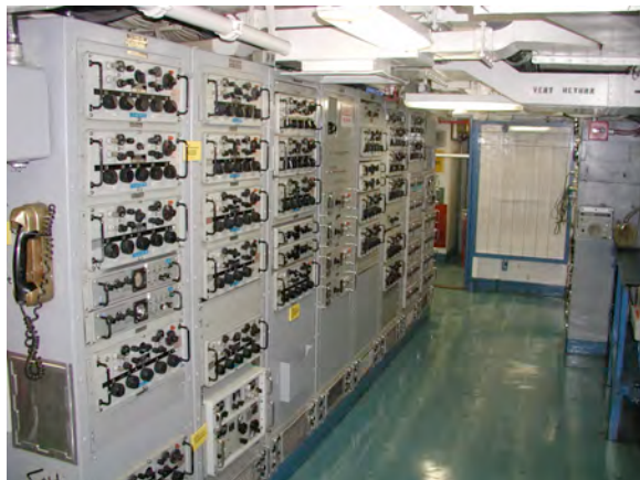
HF Receiver Cabinets (R-1051)
