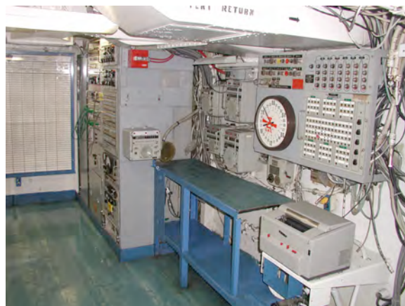
Status Board (L) & Patch Panels (R)
