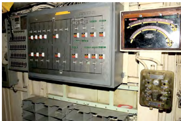
Alarm Panel (L) and Clinometer (R)
