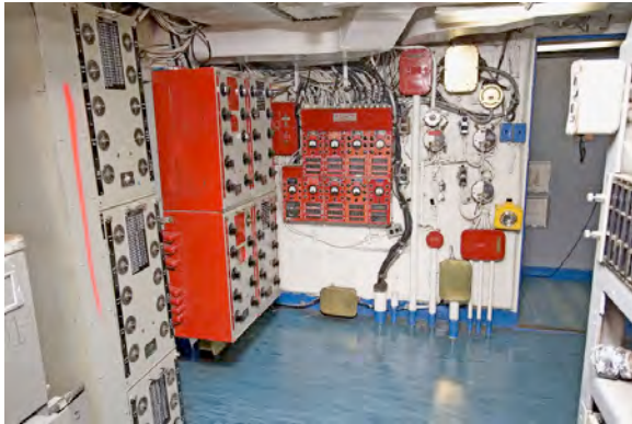
Transfer Switchboards (L) & Red DC Patch Panels (R)
