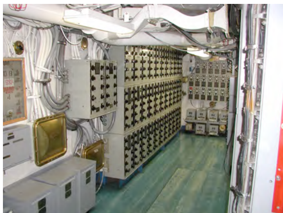
Transmitter Switchboard (SB-863) (L)
