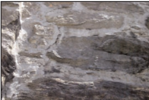
Cracks in re-pointed mortar on January 26, 2002.
