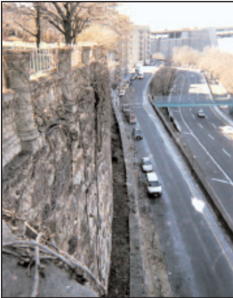
A view of pre-collapsed section looking down on Riverside Drive and Henry Hudson Parkway North.
