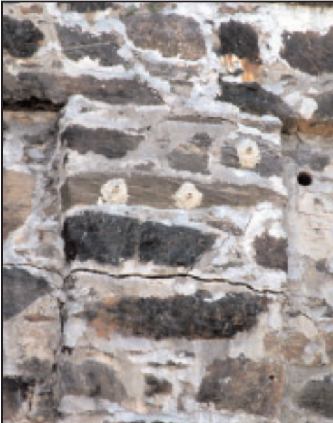
Three anchors in pilaster with large crack in lower portion.
