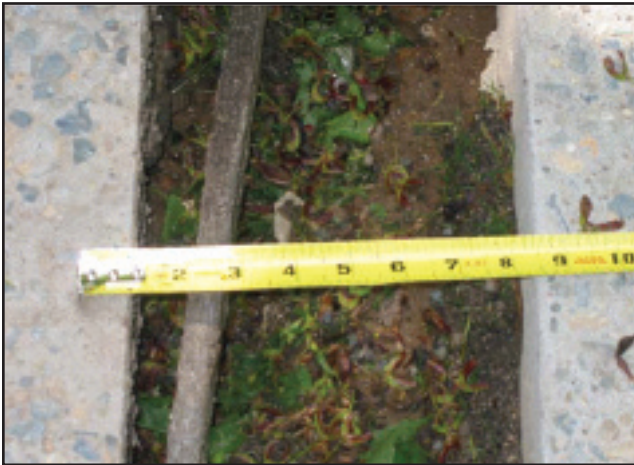
Measurement of 8 inch lateral displacement of sidewalks on May 12, 2005 prior to the collapse.
