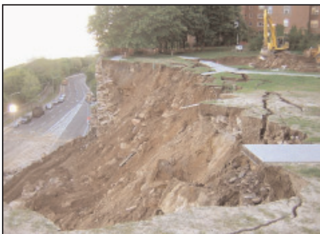
Contractors on site at collapsed portion of wall working to prevent further collapse.
