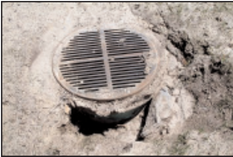
Sink hole surrounding drainage catch basin on April 19, 2005.
