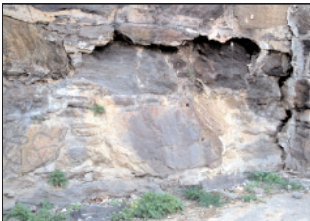
View of deformation in lower portion of wall on May 9, 2005.
