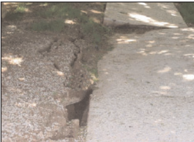
View of a sinkhole next to the park sidewalk and fissures in the park soil (both above the wall) created by the wall pulling away westward on May 12, 2005 prior to the collapse.
