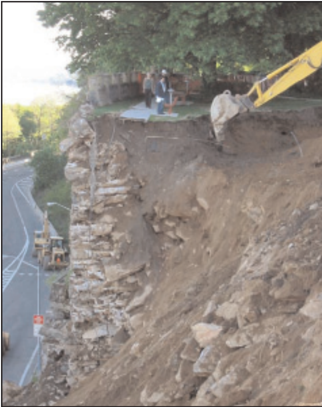
Contractors dig back top portion of collapse to prevent further sliding of debris.
