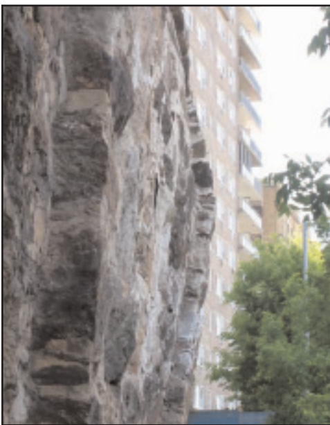
View of bowing wall on May 12, 2005.
