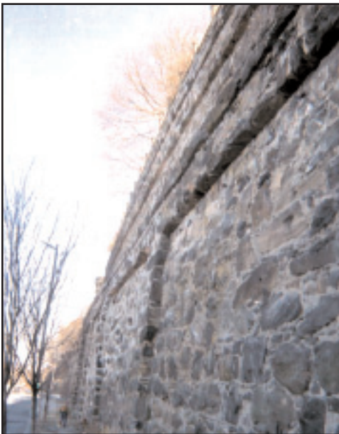
2002 picture shows curvature of wall.
