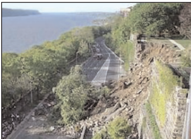
Retaining wall collapse on May 12, 2005
