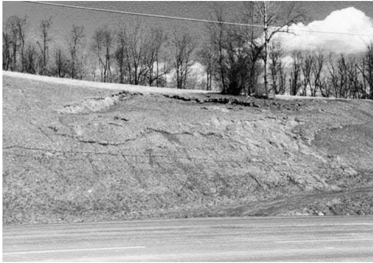
FIGURE 13.1 Slope failure near a roadway. (Courtesy of Todd Mooney)
