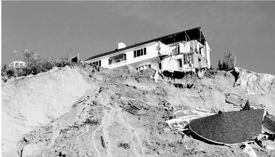
FIGURE 7.1 Shear failure of soil under a house. (© Leverett Bradley/Tony Stone Images/New York, Inc.)
