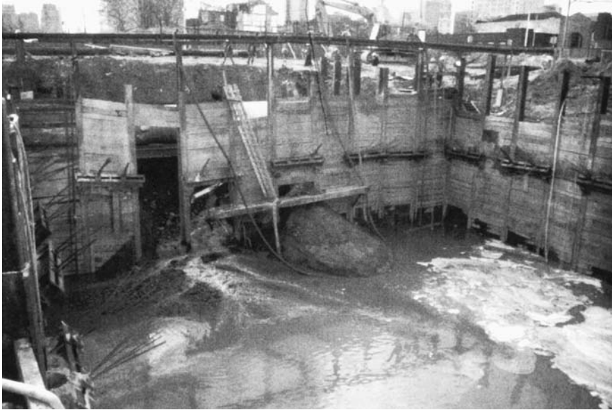
FIGURE 11.1 Damage of a braced excavation by seepage forces. (Courtesy of George Tamaro, Mueser Rutledge Consulting Engineers.)
